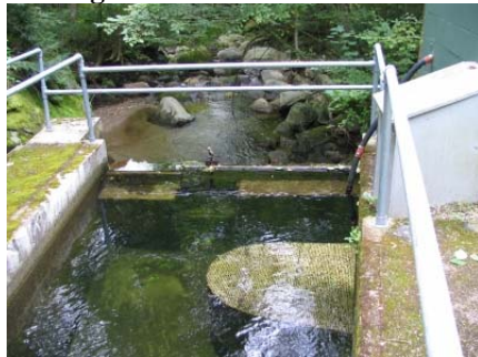
Figure 5. Kiln Brook Intake
