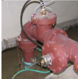
Figure 3. Field Street Wellhead
